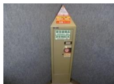
Emergency cabinet in elevators
