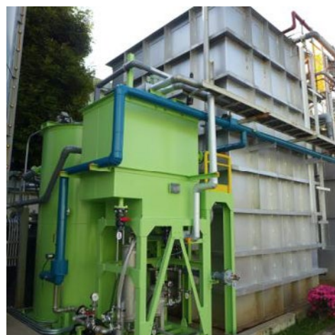
Newly installed dissolved air floatation tank (front)
