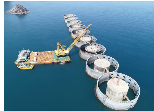
Performance retention work for main body of external breakwater (west) at Shibayama area of Shibayama Port (Hyogo pref.)
