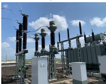
Energy facilities management
