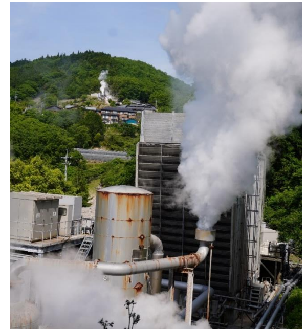
Waita First Geothermal Power Plant separately operated by Furusato Netsuden Co., Ltd.
