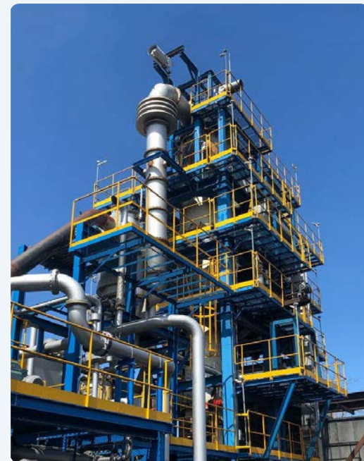
Ishikari Biomass Power Plant
