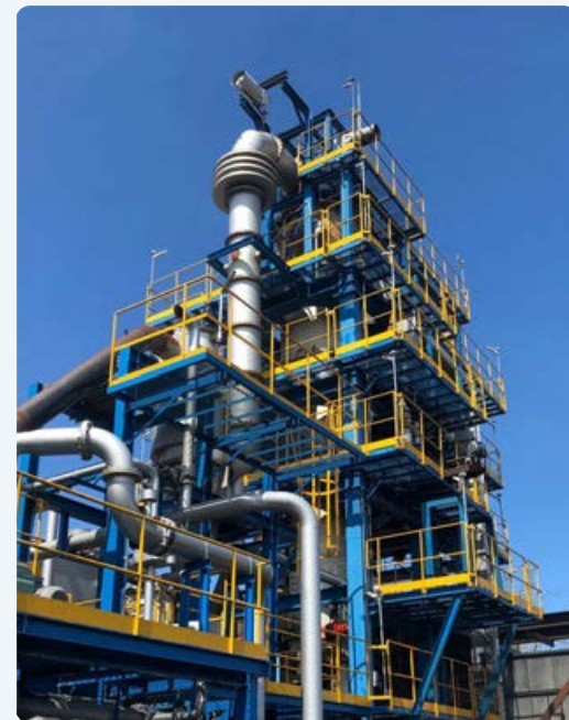
Ishikari Biomass Power Plant
